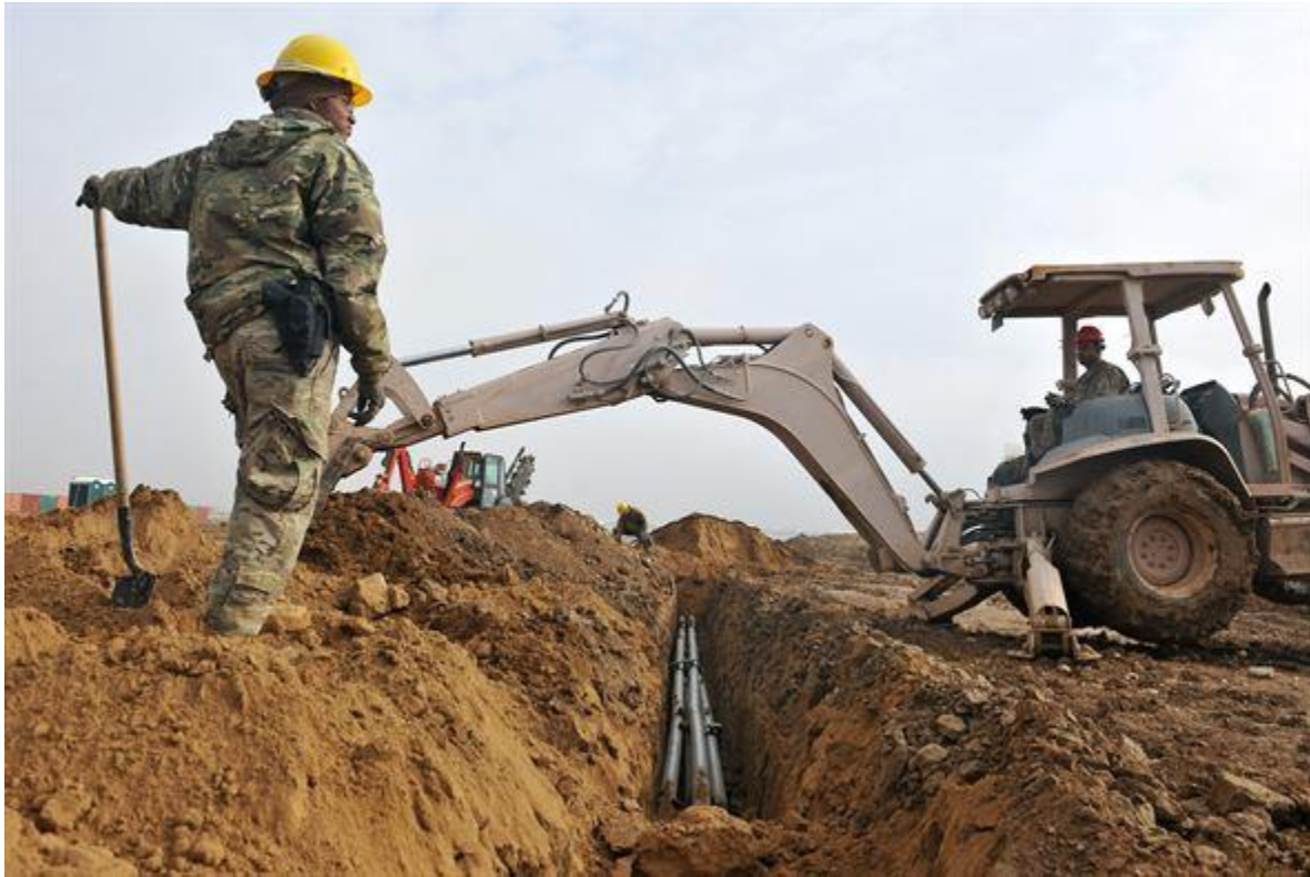
Figure 2: A direct burial fiber optic backbone for nearby Camp John Prat in Afghanistan provides a secure communication line as well as added bandwidth for web-based logistics.
